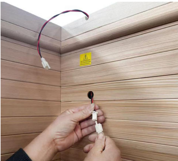
(9) Connect sauna light cable as above.
