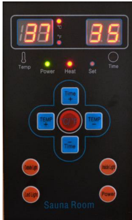
THE CONTROL PANEL
